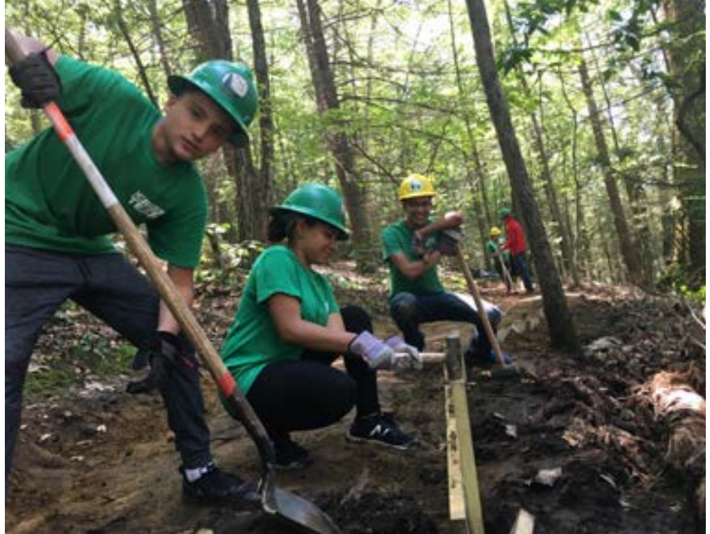
Youth from Groundwork Lawrence (MA) Green Team learn carpentry and conservation skills by building a retaining wall at the Deer Jump Reservation in Andover, MA. Photo: Groundwork Lawrence
